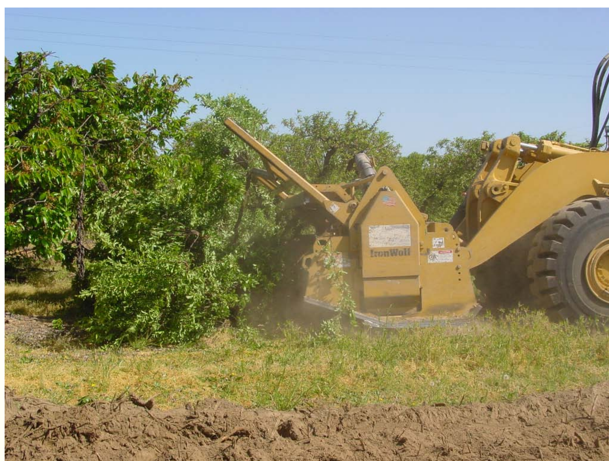
Tree being pushed over and ground in place by the 'Iron Wolf'
