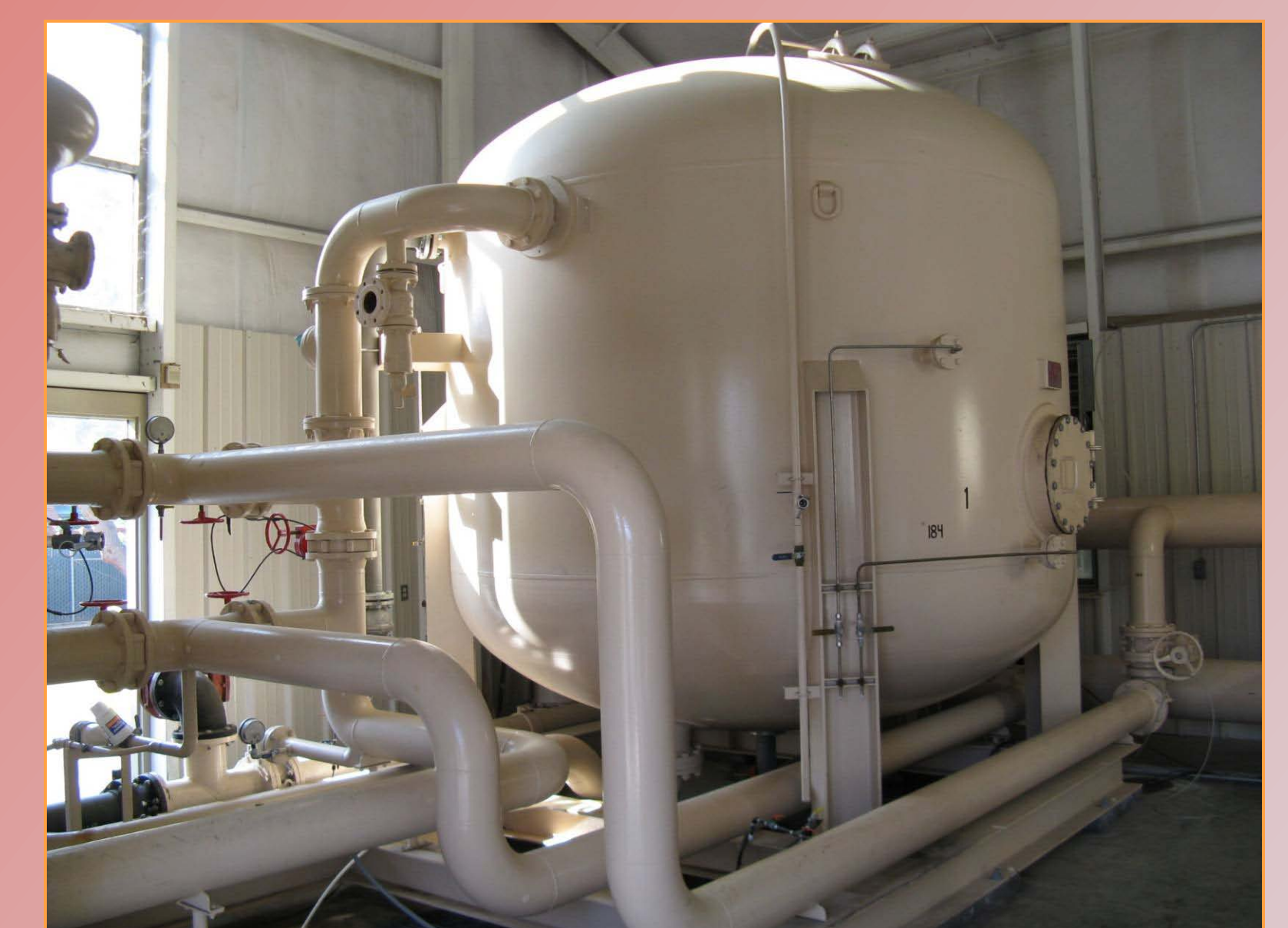
A 'Model 12' vessel filled with 740 ft 3 of GAC for DBCP removal. Almond shell GAC filter columns will be installed at the inflow to this vessel.
