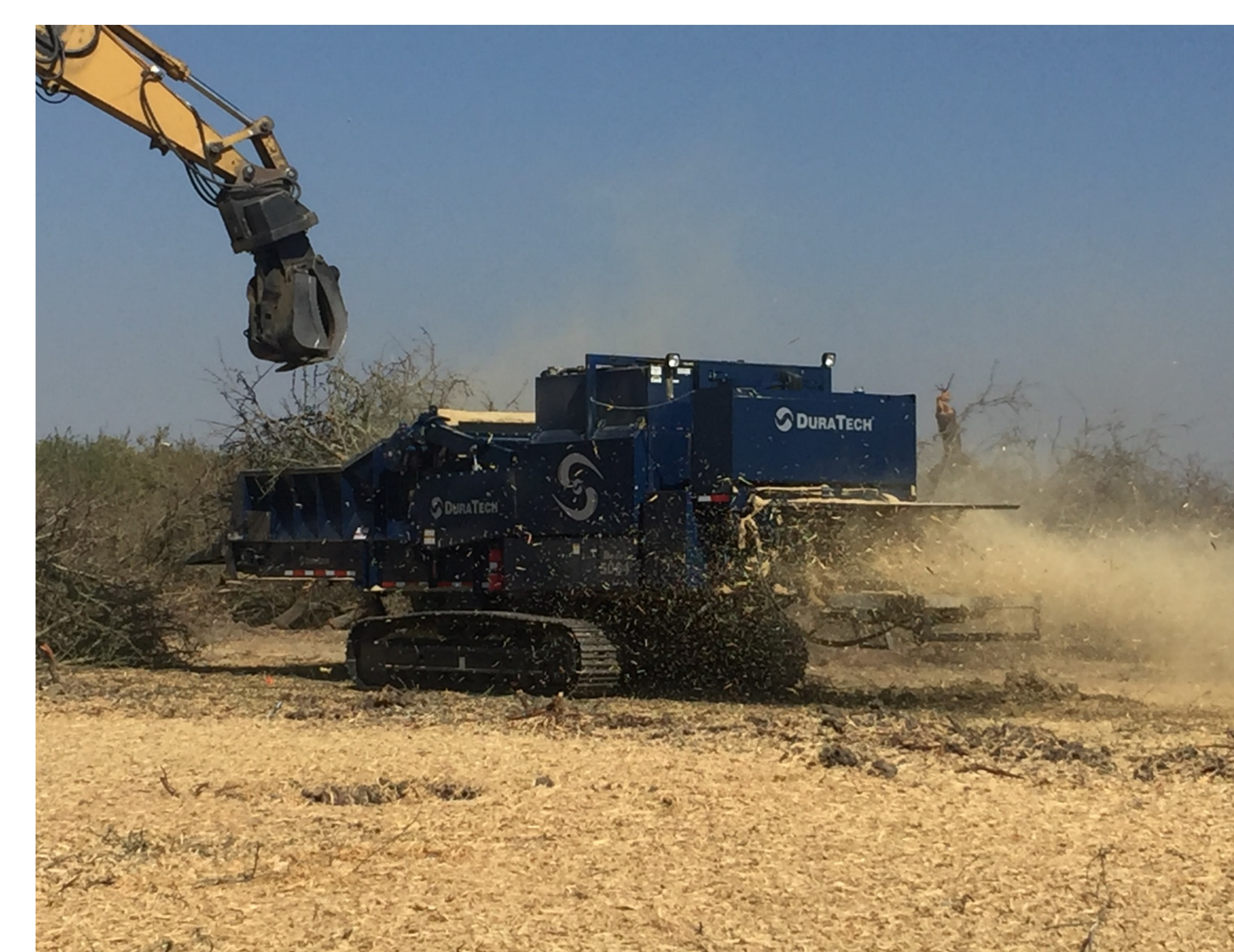
Figure 7. This Duratech grinder is mobile and spreads the wood chips evenly as it grinds.
