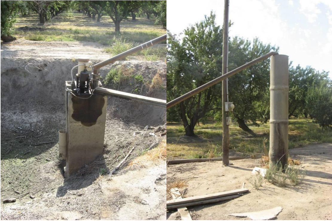
Figure 6. Recirculation Pump and Stand Pipe at South Side of Basin
